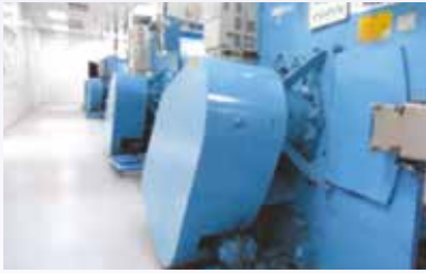
De-Ionized Water Wash ISO 5 Cleanroom
